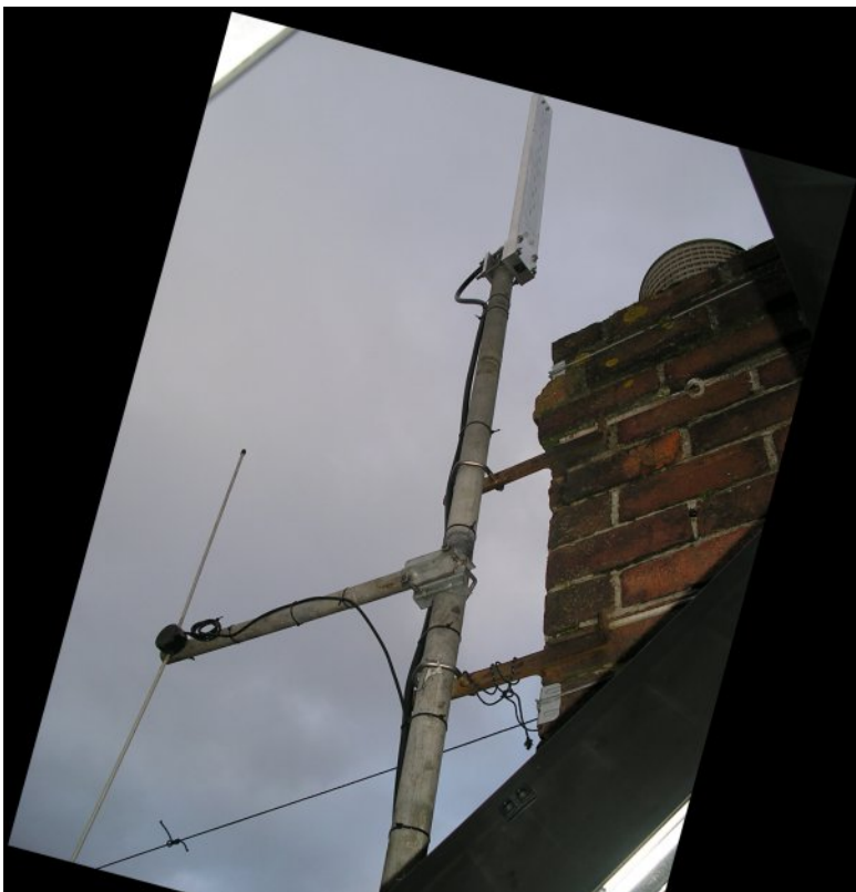
The 3.4GHz slot (for GB3FB) and the vertical dipole for 144.750MHz DTMF control
