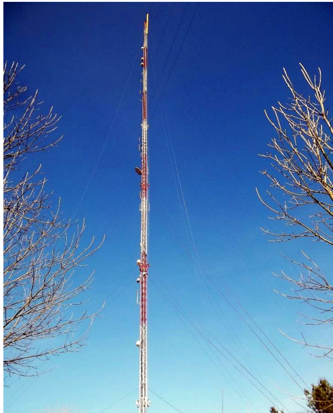
The tower with the gin pole at the top. It's the yellow item clamped to the 1065' tower side ready for the new antenna
